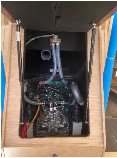
Compact – Poor ventilation
